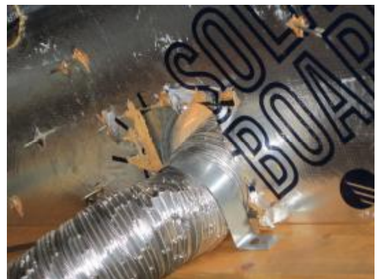
Possible point of entry.
