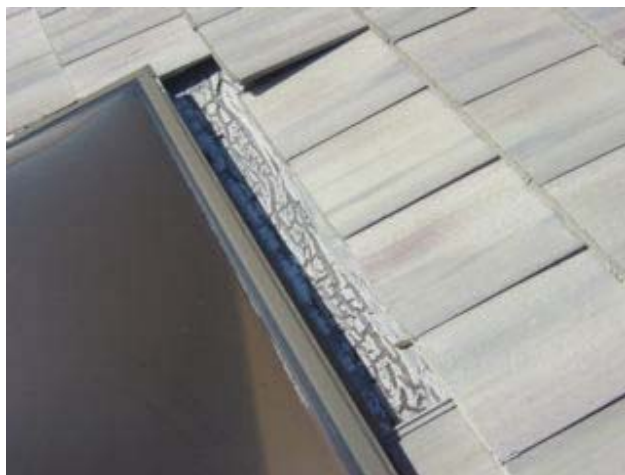
Picture 5: Reseal seam above skylight.
