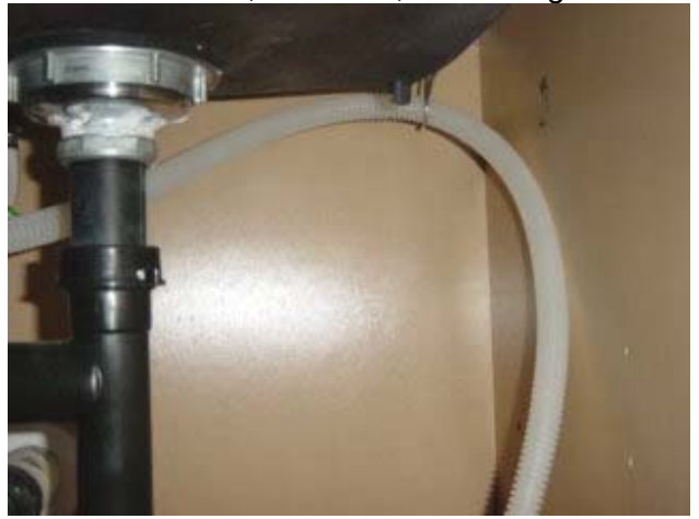
Picture 9: Waste drain hose from the dishwasher.
