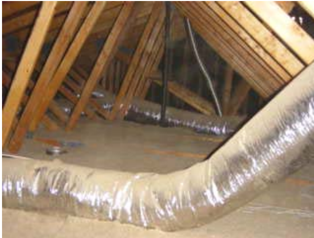
Picture 8: Ducts not hanging from trusses.
