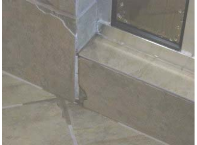
Picture 10: Leak base of master shower.
