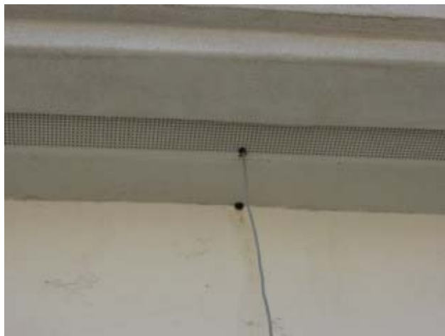
Picture 1: Holes in soffit east side of house.
