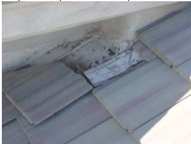
Picture 4: Tile slipped out of position, east side of covered entry.
