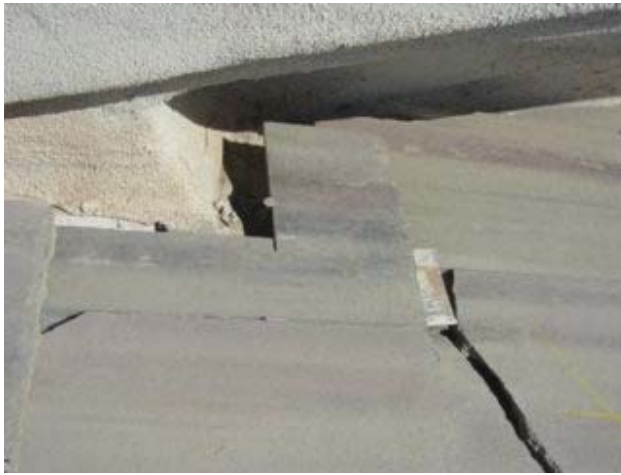
Picture 7: Poor transition between tile and wall west side of entry.
