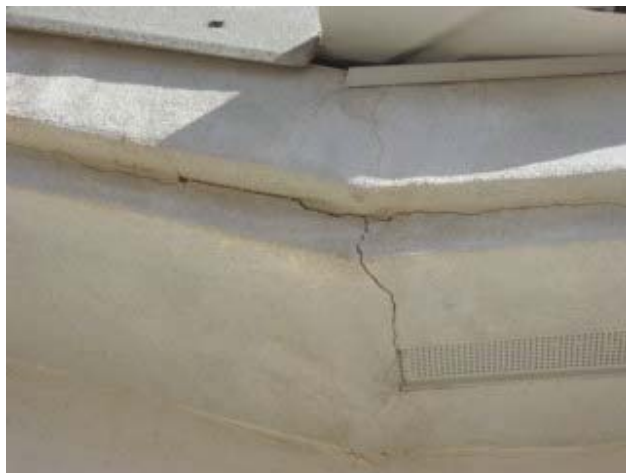
Picture 2: Cracks in stucco on soffit west side.
