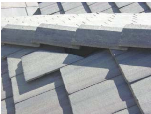
Picture 6: Example of tile slipped at hip.
